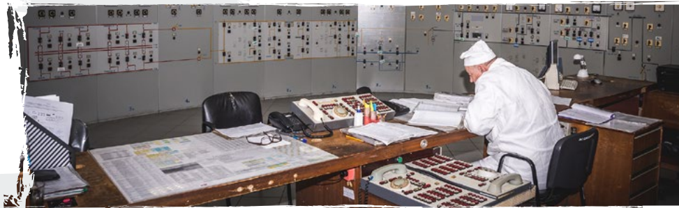
CENTRAL CONTROL ROOM
