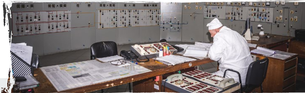
CENTRAL CONTROL ROOM
